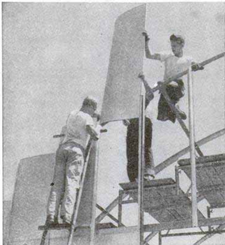
Frame of aluminum building is assembled on ground. Below, flanged sheets slip into frame to form the walls
