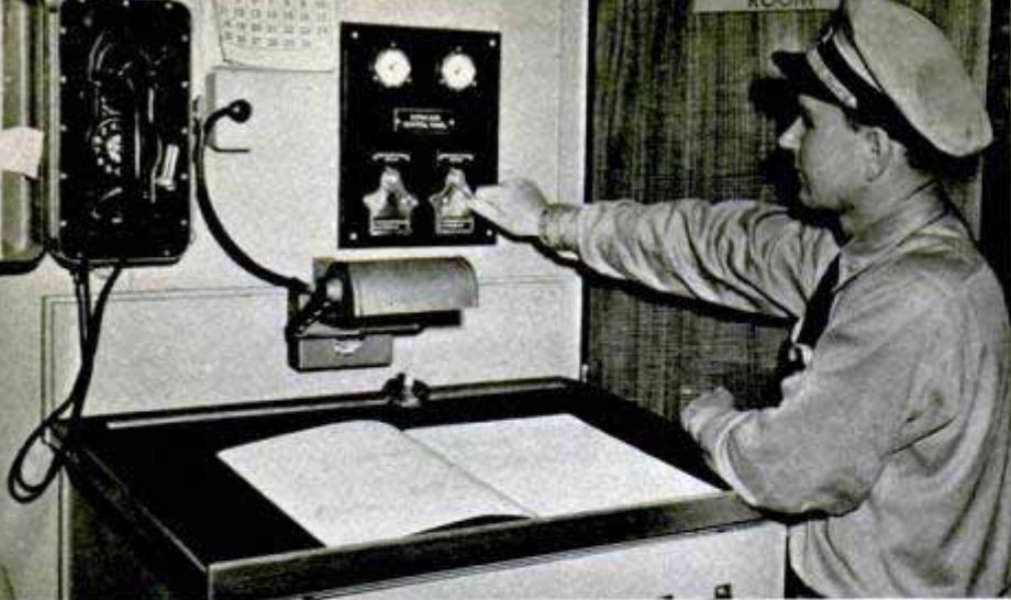
Alarm system sounds a warning in fire-control room (above) when automatic devices detect smoke or flame in any part of the ship
