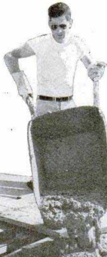
Sawdust-concrete, though of coarse texture, spreads very easily. Here, workmen cover reinforced wire mesh with a thick coat of the mixture to form the solid floor slab
