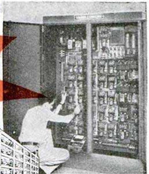
Student trouble-shooting large control panel in school shops.
