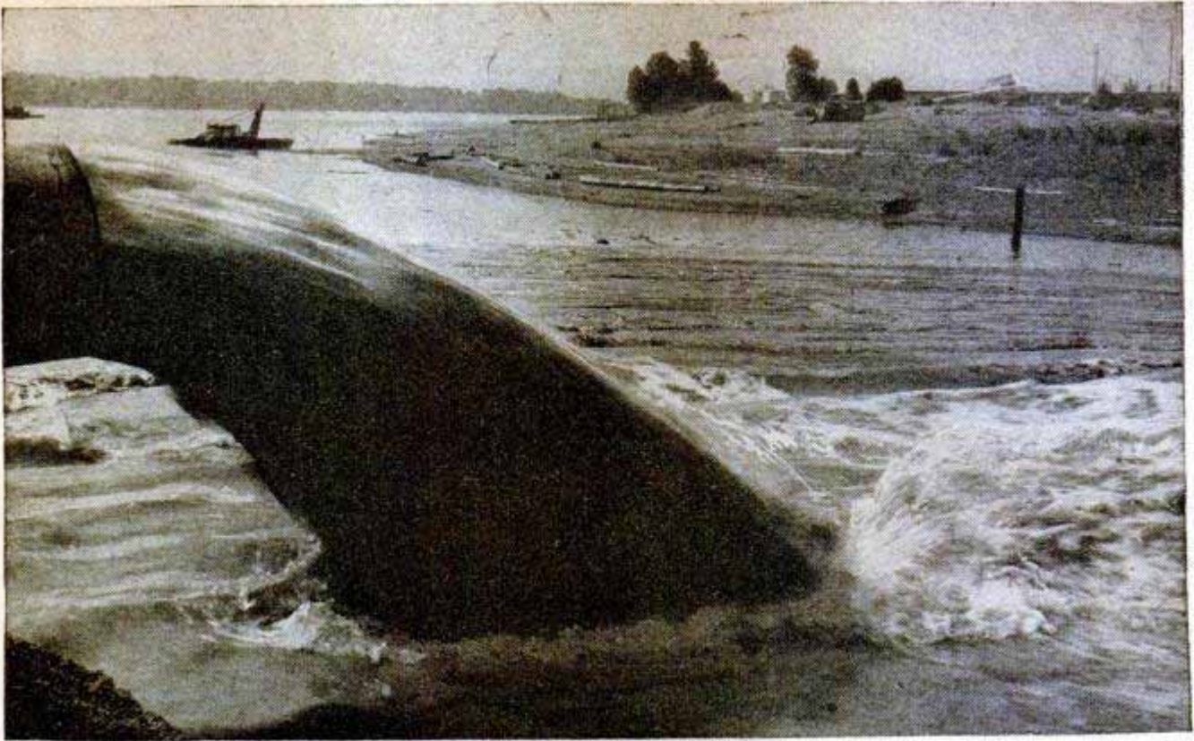
From the suction dredge's 24-inch discharge pipe pours a torrent of sand-laden water
