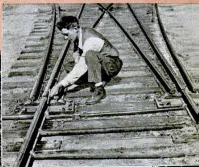
Switchman below checks clearance of an ancient stub switch. At bottom, after switch is thrown the engineer of oncoming train is waved through
