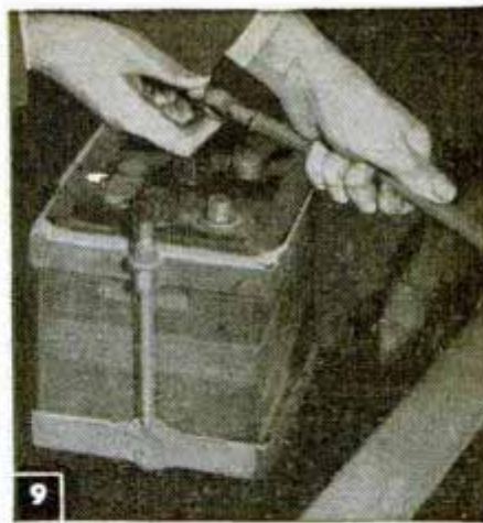
9 Worn or frayed cable should be replaced. Note bends in old cable and install new one in the same way
