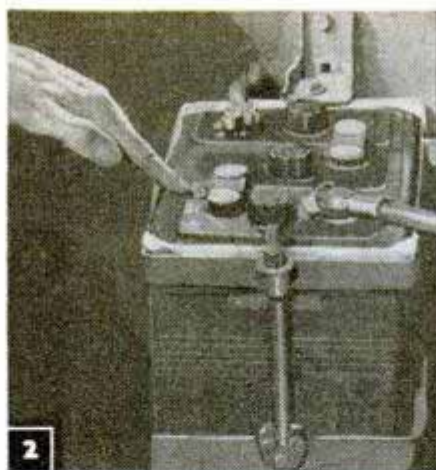
2 Check sealing compound for cracks. Repair with compound, using in a tarry consistency that does not run
