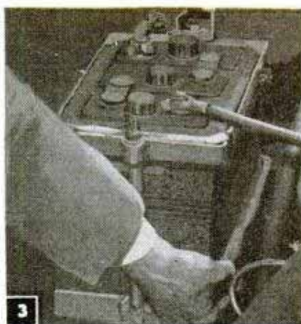
3 Inspect the battery cradle for acid damage. If the cradle is in poor condition it should be replaced
