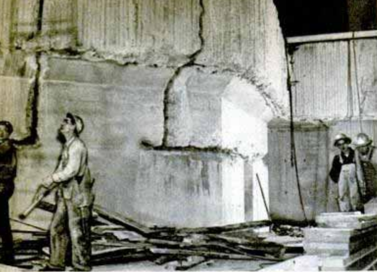
Concrete is chipped from massive generator at Grand Coulee so the power unit can be moved to Shasta Dam
