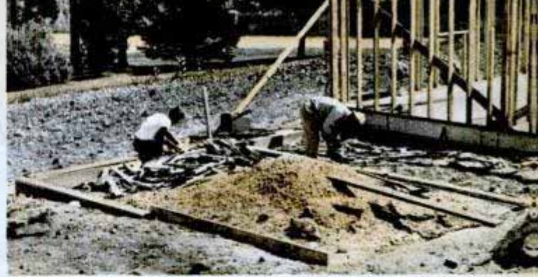
After erecting the studs for the main part of the house, put up those for the garage and bridge across the breezeway to support ceiling joists
