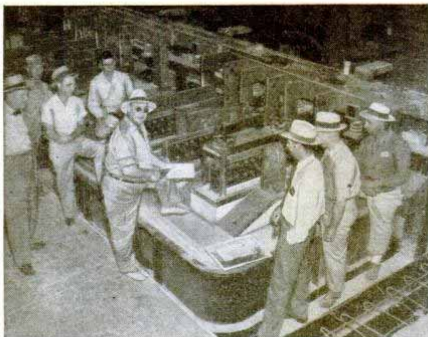
At Basic Magnesium Plant, Las Vegas, Nev., bus bars (background) connect to electrolytic cells (foreground) where magnesium was "cooked"
