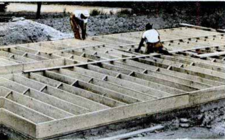
Floor joists are next. These meet and overlap at the center member. They are laid on a wide sill which is bolted to the concrete foundation wall
