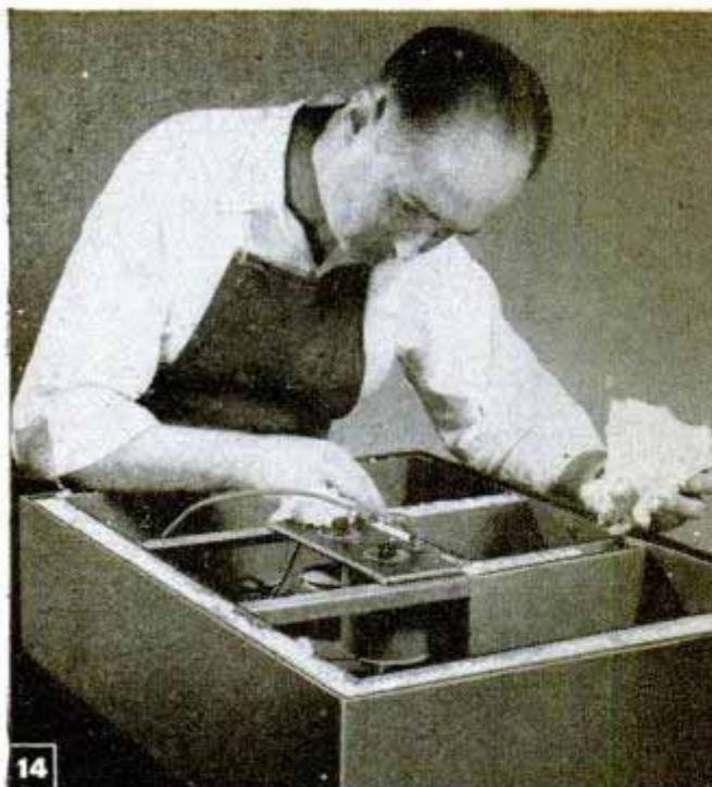
Packing insulating material between walls of unit. Insulation is covered with strips of hard-pressed board
