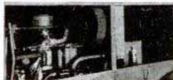
POWER PLANT Left-Side Interior View
