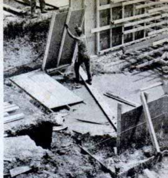
JUNE 24 —"Bud helped set forms for the foundation. Also laid some sewer tile"
