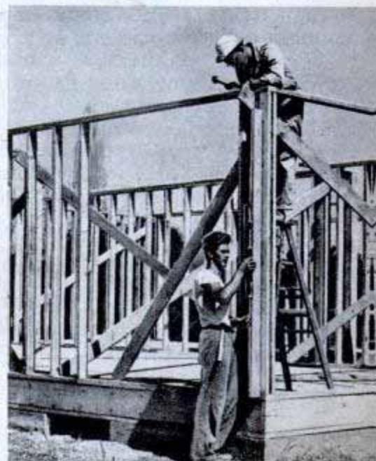
↓ JULY 12 —"Bud and I put in eight hours each raising framework. Is my arm sore!"
