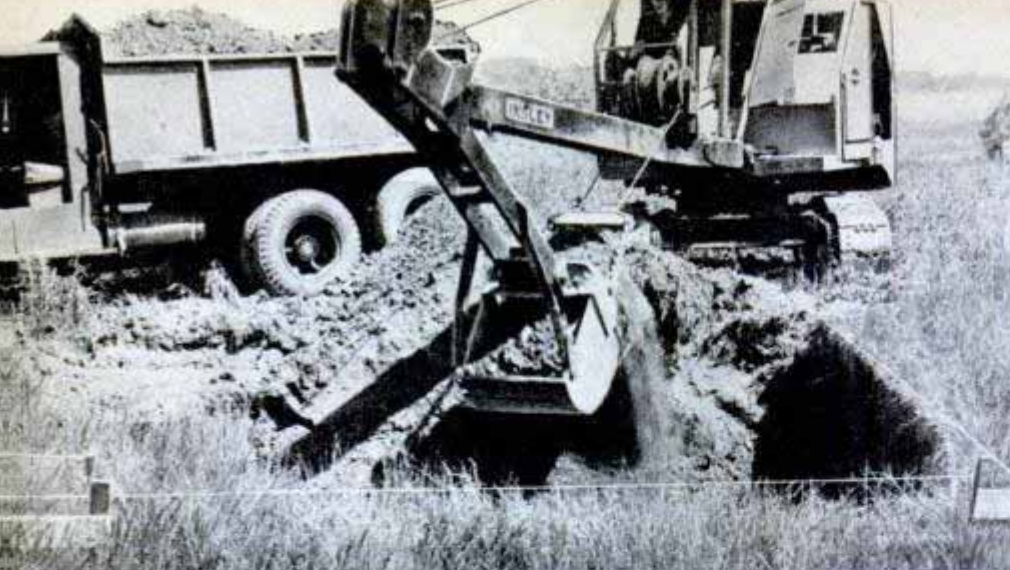
MAY 29 —"Big day for us. Ground broken for house and excavation well under way. Removed 200 yards fill dirt. Trucking cost $30"
