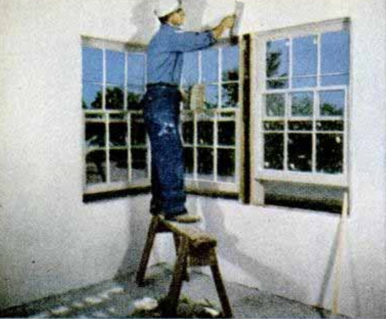
Jacques adds finishing touch to the plastering, one of the few jobs requiring expert assistance
