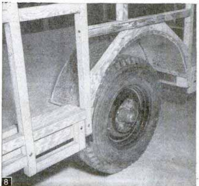
8 The sheet-metal fenders are carried down below the floor line to prevent water from seeping in onto floor
