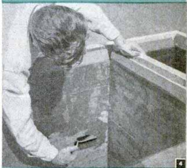
Here the final coating which forms a seal between the sheet metal and the cork is applied
