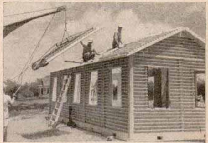
Roof section is added. House has a ceiling ventilator which circulates air in all rooms and closets
