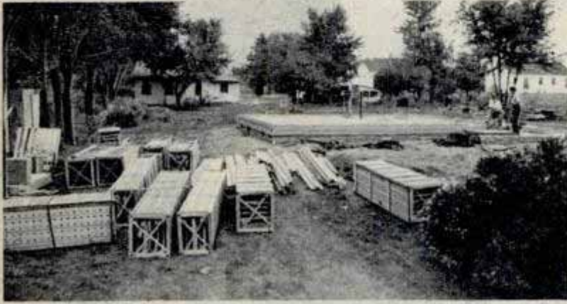
Aluminum panels for the house walls and roof arrive at the building site in shipping crates. Below, in two days three fourths of the house walls are up as are the walls and girders for garage
