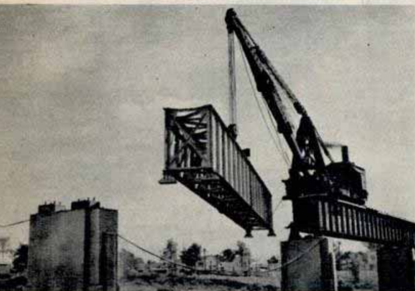
First all-aluminum bridge span swings into place across Brasse River at Massena, N. Y. It weighs 53,000 pounds. Same size steel span weighs 128,000 pounds
