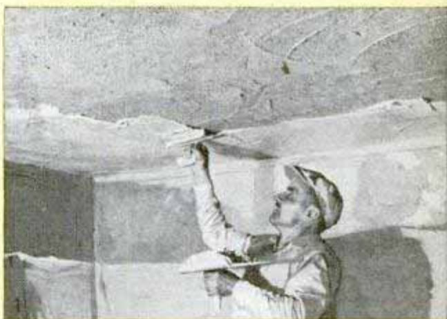
Second coat is applied 1/4 in. thick when the first is thoroughly dry. It should be pressed in to adhere to the rough surface of the first coat. For a three-coat job, second coat also is roughened
