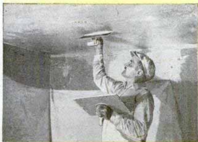
The final or "setting" coat should be 1/8 in. thick. It is applied when the second coat is nearly dry, but not too dry or the moisture will be drawn from the mixture, making it difficult to trowel
