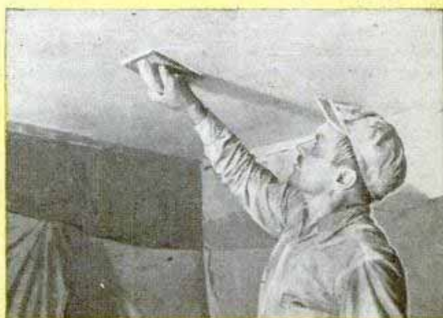
Final coat may be troweled to a hard finish, or it may be given the "sand-float" finish shown. This is done with a wooden trowel in a circular motion (Photographs courtesy U. S. Gypsum Company)
