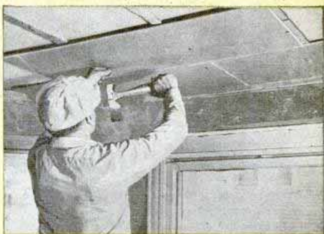
Next, plasterboard is nailed to the strips to form a smooth surface to which the new plaster will bond tightly. Place the sheets so that the joints are staggered and meet on centers at the strips
