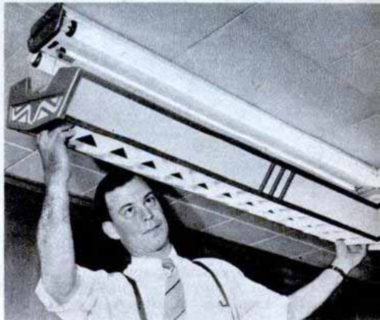
Chain arrangement on fluorescent light fixture permits lowering lamp enclosure and supports it while it is being cleaned. Chains unlock for complete removal
