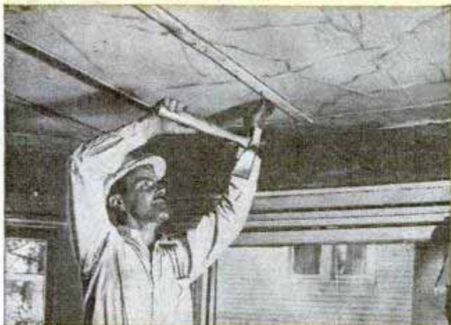
First step in renewing a badly cracked or sagging ceiling is to locate the joists and cover them with furring strips of lath, nailing the strips over the old surface in line with the joists
