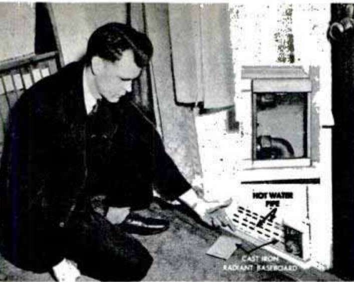
Radiant baseboards made of hollow cast iron distribute hot water heat evenly throughout a home
