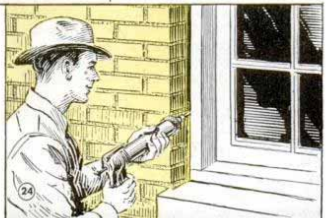
Window frames in old brick homes must be recaulked before painting. Be sure that the cracks are filled flush with the surface
