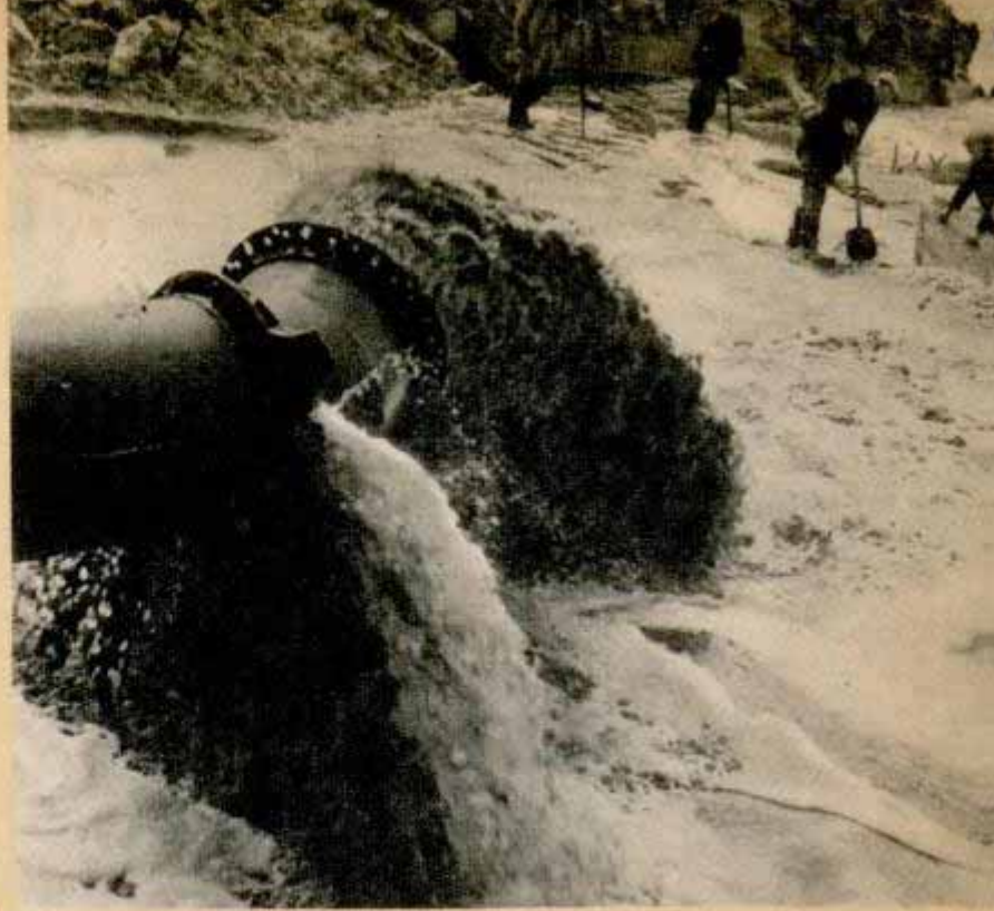
Above, a thousand tons of sand pour through giant pipe each hour to form core of dike. Left, huge dredge drops antisubmarine net and scrap into German barge that was sunk to seal final gap successfully
