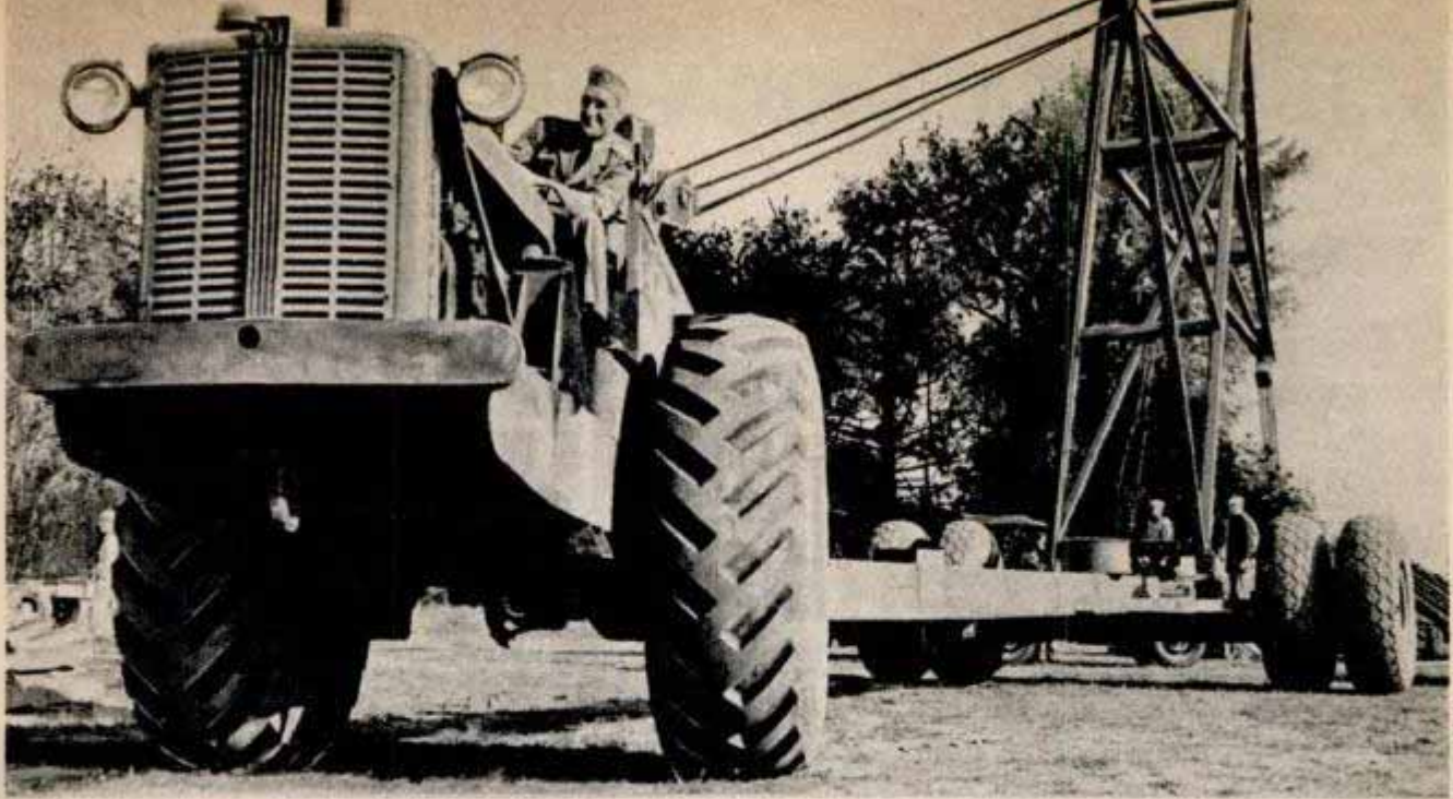
CRASH TRUCK originally built to salvage wrecked bombers and fighter planes was put to work laying gasoline burner pipes along the edges of an airfield at Arcata, Calif., in connection with FIDO fog-lifting equipment
