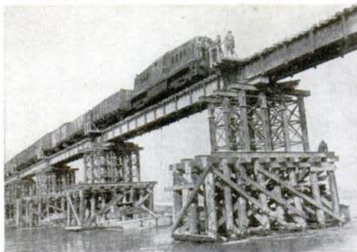
U. S. Army engineers built this bridge across the Rhine at Wesel, Germany, in just 10 days. Below, looking into steel piling cofferdam as concrete is placed for pier of Santa Fe's new Colorado River bridge
