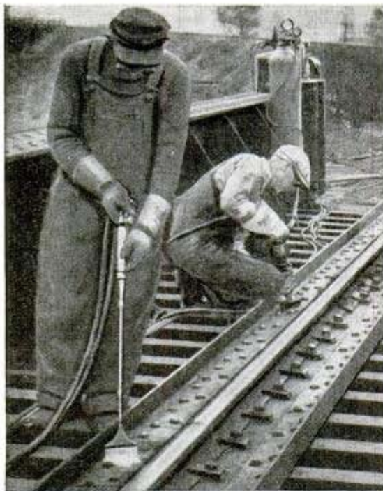
To guard against rust, old paint is seared with multiple-burner torch and removed with a power-driven brush that leaves surface clean for fresh coating Oxweld Railroad Service Co. photos
