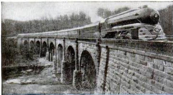
112-year-old stone bridge at Relay, Md., carries heaviest B & O rolling stock. Engineers say it will last for centuries
