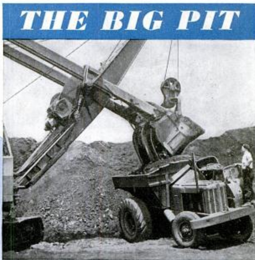
Electric shovel loads iron ore into small "Dumpton" at Spruce open pit near Eveleth, Minn. Below, around the Big Pit iron ore trains run on terraces at different levels removing ore and waste material
