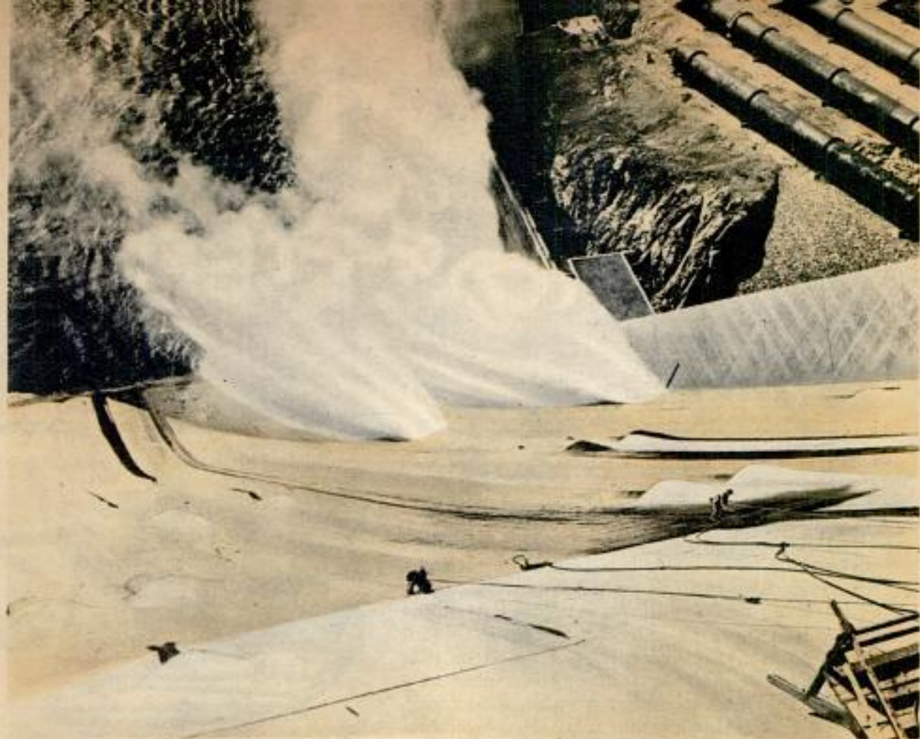
Workmen caulk spillway seams of Shasta Dam. Pipes 15 feet in diameter, upper right, supply generator units
