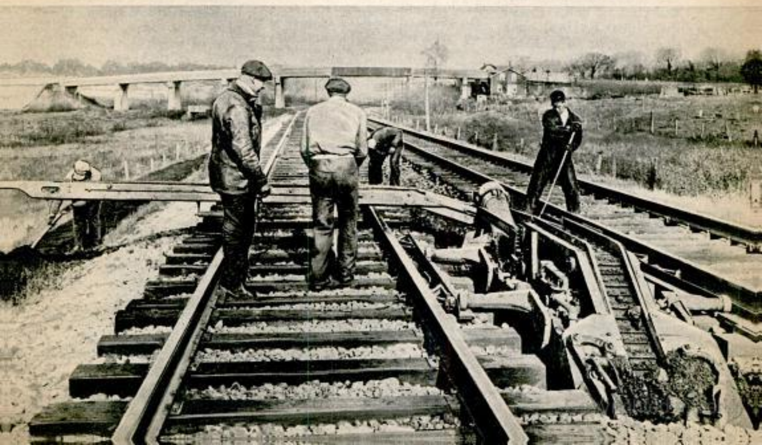
Another type of ballast cleaner moves along edge or center of ballast, deposits dirt along right-of-way Bessemer & Lake Erie photo
