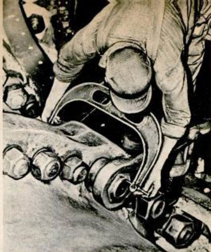
Micrometer measures stretch of one of a thousand bolts holding case of Grand Coulee 150,000 hp. hydro-turbine
