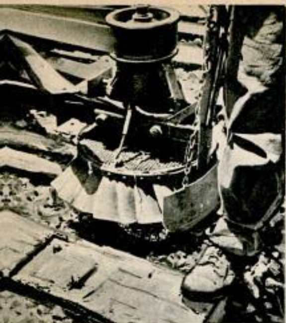
Screen and flaps of power adze above keep chips from flying up. Cleaner for ballast, right, ejects dirt and cinders
