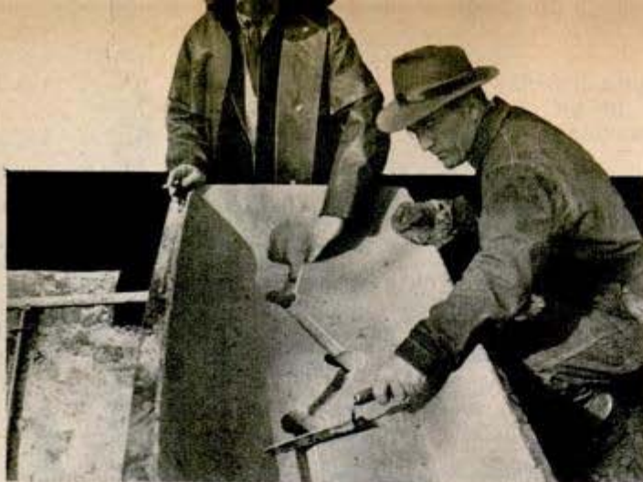
Mold box with pouring gates located at each end is built over each joint to be welded; hot steel is poured in this basin and funneled into gaps between ends of castings. Below, a portable crucible filled with aluminum particles and iron scale gets ignition charge
