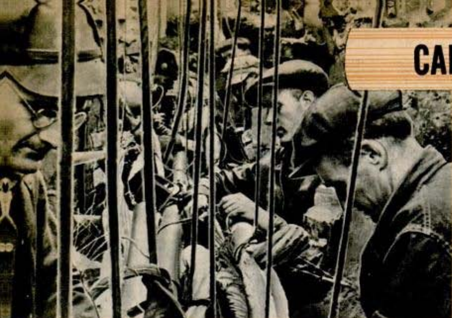
Jobs like this—splicing badly damaged telephone cables—provided civilian workers with practical know-how which helped our Army cross Europe
