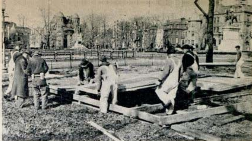
Even the floor of "blitz" bungalow is laid in sections. Here a sample house designed for Allies is being erected in Washington, D. C., park
