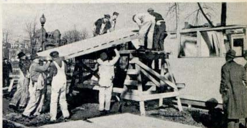
Above, workmen raise first of eight roof panels to proper level. Panelized construction makes job of assembly easy for unskilled workers
