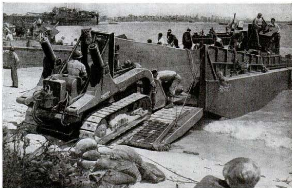
Bulldozer runs up on ramp to help unload LCM landing on Pacific beach. LCMs had major role on the Rhine
