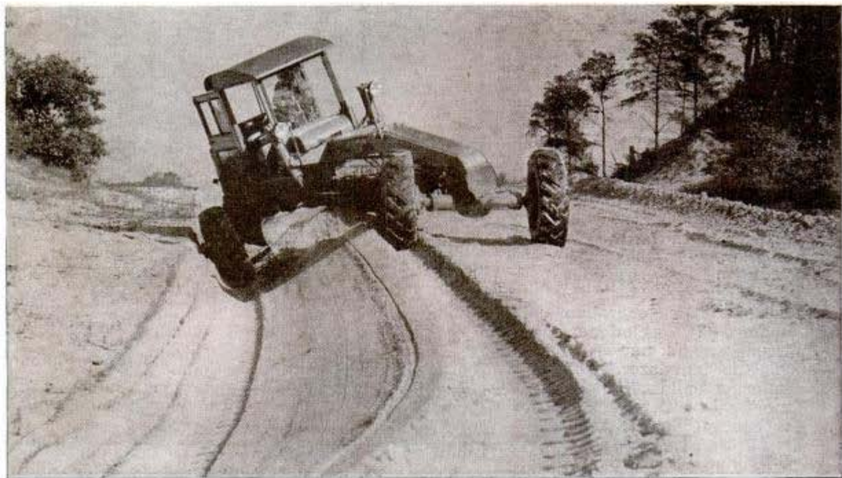
Ditch-digging, too. Preliminary to deepening ditch, this Austin-Western moves windrow from shoulder line
