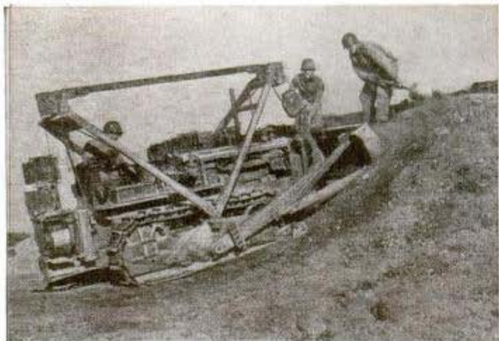
When airport building boomed after landings in North Africa, the bulldozers found plenty to do. Above, "Cat" throws up a revetment
