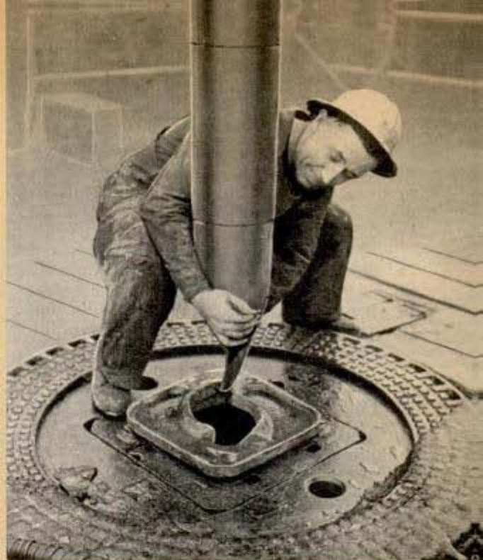
Top left, examining the bit that cuts through the rock to drill hole thousands of feet deep. Fast-drilling "fishtail" bit (above) is used until hard formation requires rock bit. Bottom, lifting a long section of pipe from a hole
