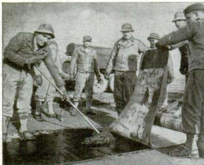
Above, the underside of P.H.S. Note black surface showing that the asphalt coating has been cut back. A new roll of P.H.S. is being started
