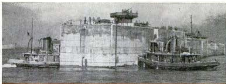
Tugs jostle the concrete caissons into position. Note anti-aircraft gun mounted amidships. Below, aerial view before storm wrecked harbor
