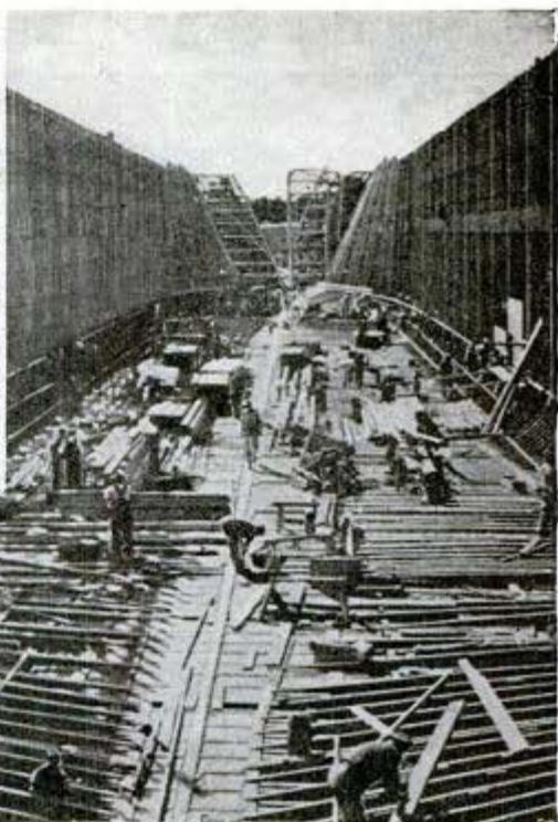
Above, a wooden form resembling the skeleton of a prehistoric monster is built to set the ship's contours and hold the reinforcing steel in place
