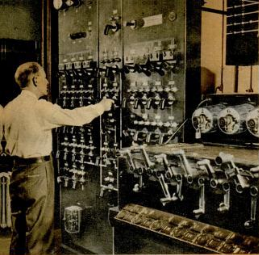
Operating the remote-control circuit breaker on control panel in Union Tower at Rahway, N. J., for nearby power station
