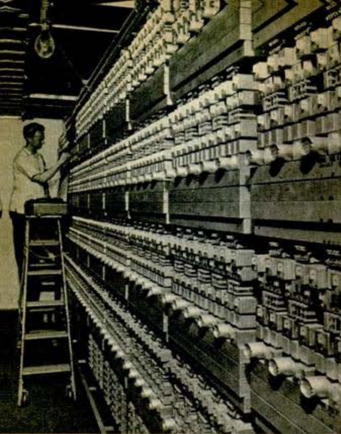
Western Electric photo Adjusting relays (in which large quantities of silver are used) in Navy telephone switchboard
