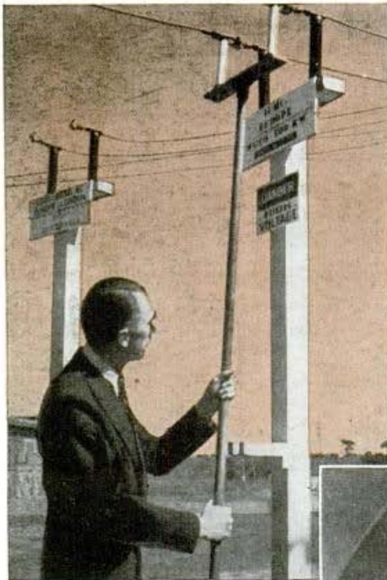
In the "switchyard" of a short-wave station a program is beamed to Europe
