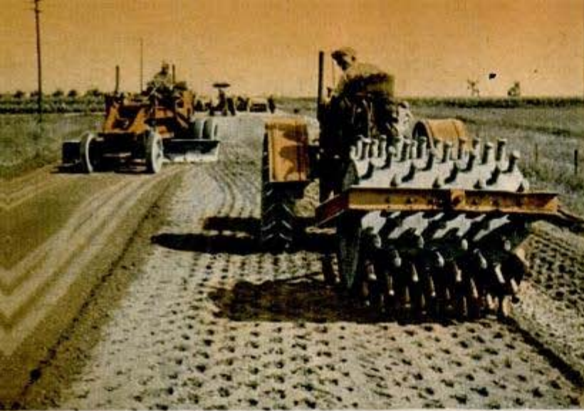
Strip of soil-cement highway gets a final sheepfoot rolling and smoothing with scraper. It forms smooth hard-packed road
