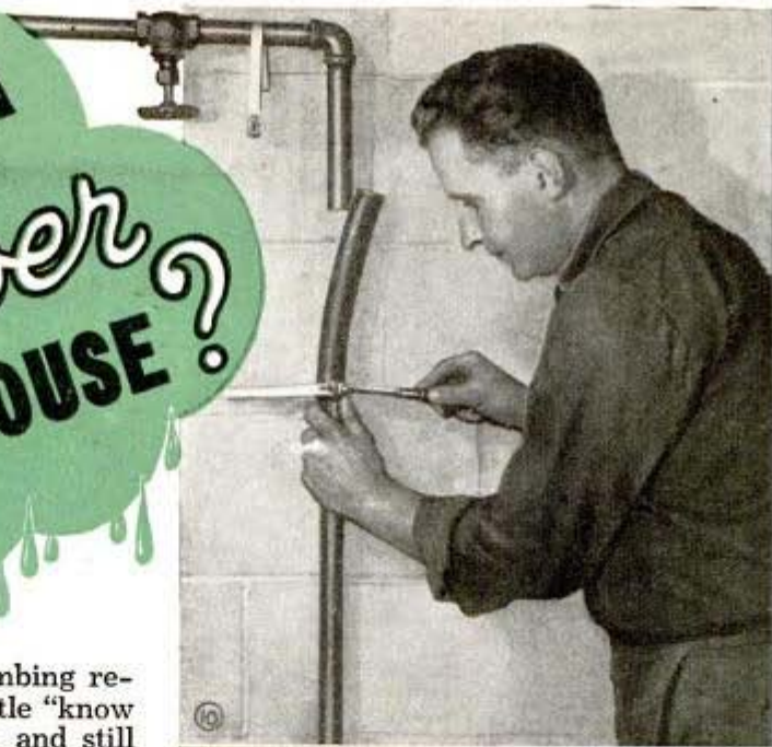
PIPE LEAKS can be repaired permanently with rubber hose, as shown above. Other temporary methods are shown below together with table for determining length of pipe replacements
