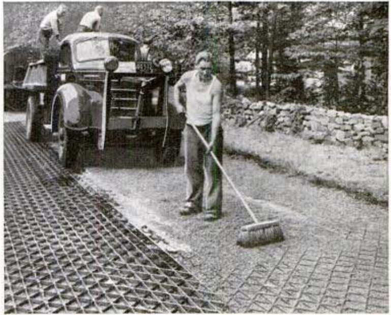
Landing-mat type of steel grating is laid for test roadway and graveled
