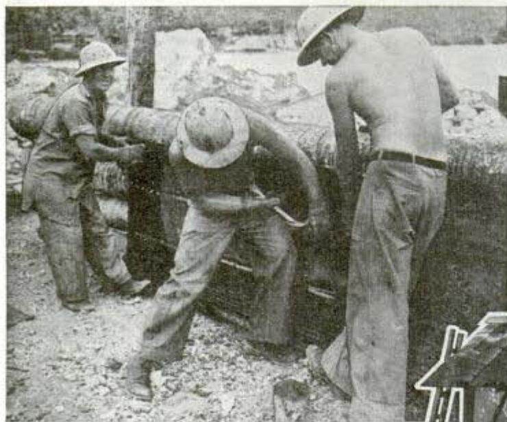
Classic examples of American ingenuity at work are found in the way the Seabees, the Navy's Construction Battalions, use empty gasoline drums as building materials. Either intact or flattened, the drums are prized for construction. Left, shoring up a dock with some flattened drums
