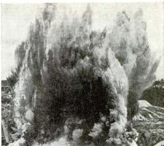
Here's what 50 tons of dynamite, going up at once, look like. Blast removed 18,000 yards of rock, and was felt 50 miles away
