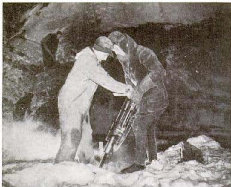
Inside one of six great tubes leading to powerhouse, members of ice crew use pneumatic hammer on ice so diggers, muckers, blasters can get to work
