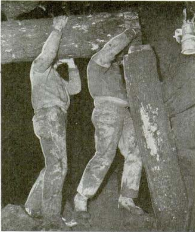
Raising an 18-inch cap timber in a tunnel of the Mouat mine
