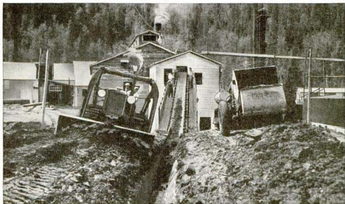
Bulldozer shoving rich oil sand onto long conveyor belt which carries it into the plant's oil separator
