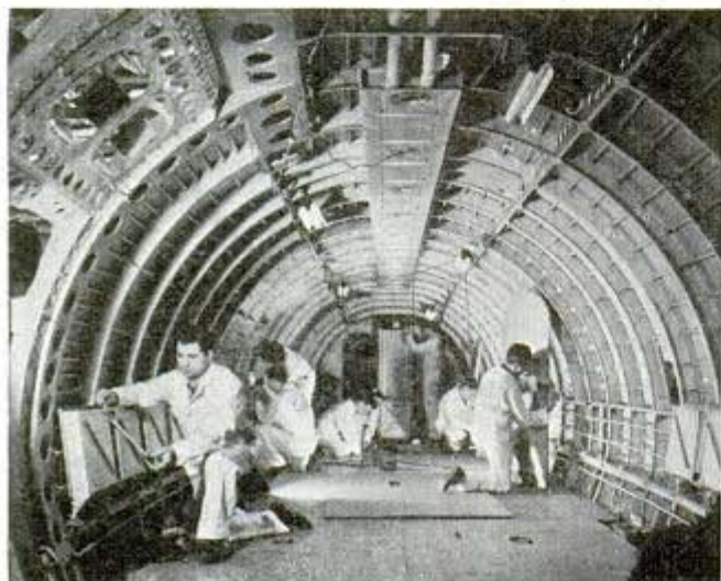
This view of the inside of cargo plane under construction gives some idea of its size; the workmen are installing folding seats
