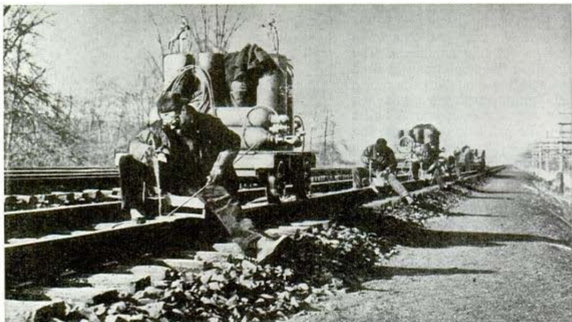
Building up worn rails by oxy-acetylene welding helps carry increased war load with safety and speed. Some defects are caused by continued pounding at joints where roadbeds are weak
