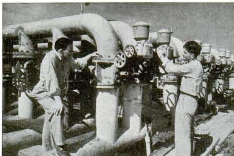
Various forms of crude oil flow through these pipe-line manifolds to refinery for cracking
