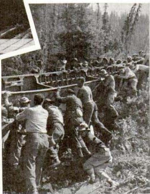
In battle against wilderness, the engineers building Alaska highway launch ponton which will help to support a bridge. They have conquered many a nameless stream between Fort St. John, Canada, and Fairbanks, Alaska
