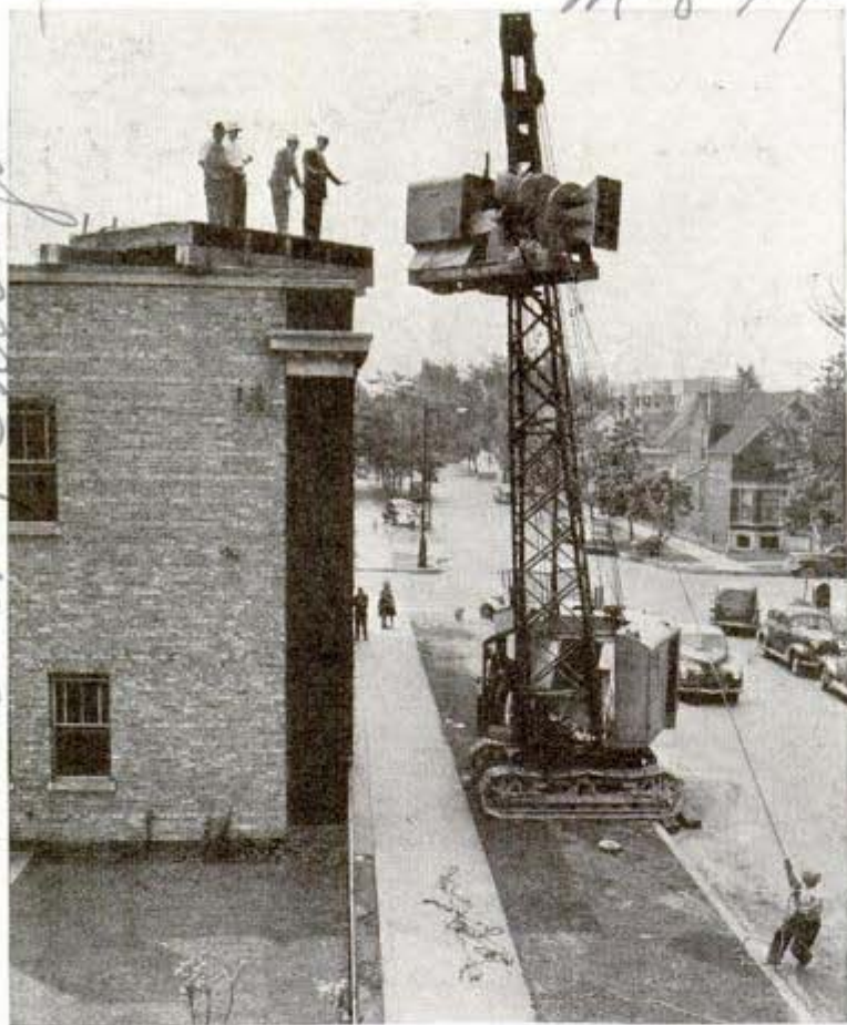
Lifting one of Chicago's 5,000-pound air raid sirens to roof of fire station. Twenty of the sirens, audible nine miles away, are being installed
