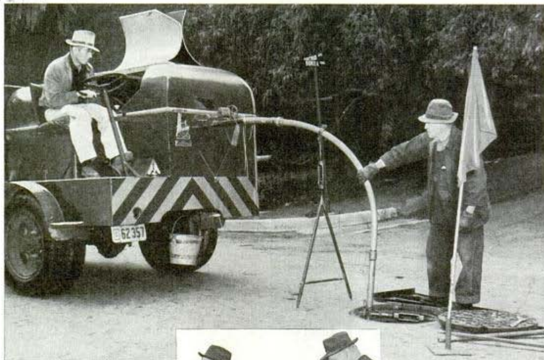
Operating a power sweep that feeds cable down the curved pipe to move a cleaning rod
