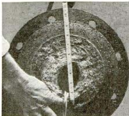
This eight-inch pipe was nearly clogged with a thick coating of industrial waste
