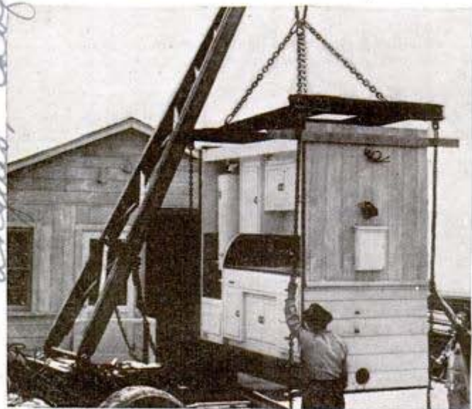
Ready-made kitchen and bath unit, being hoisted from truck, may be installed before or after the house has been erected
