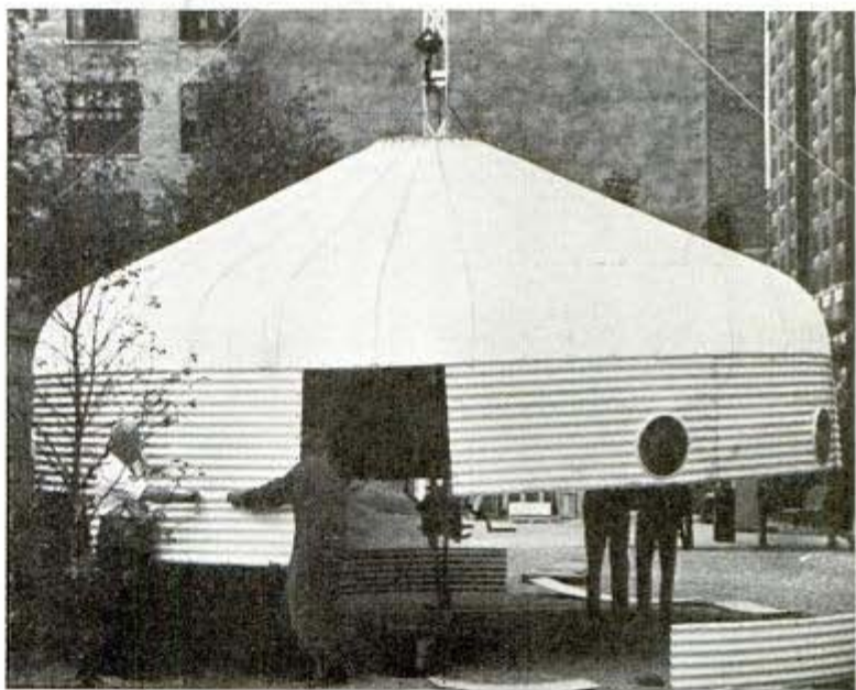
Another view of the circular metal house showing the roof being lifted on the steel mast and some of the wall sections bolted in position
