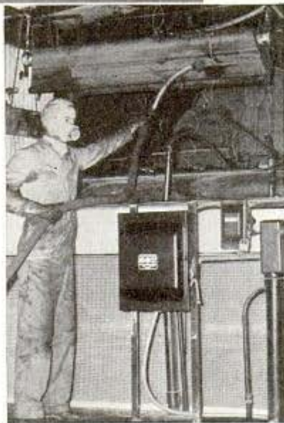
Testing a fluorescent light fixture to be used in factory with a dust hazard
