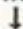
This is another view of the metal-clad rotary converter with which a chemical factory translates its "a.c." electricity into direct current for producing a vital element of aviation gasoline. The metal trailer-shaped housing prevents chemical fumes from reaching the converter
