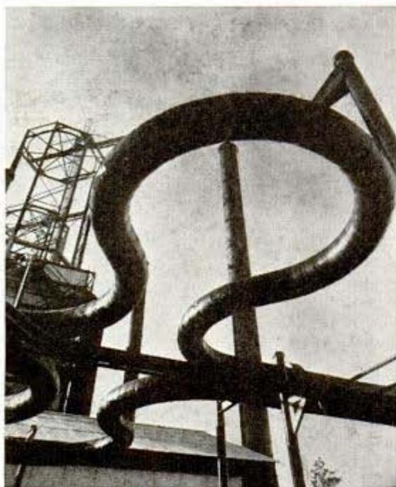
Expansion loops in hot oil lines at a big refinery
