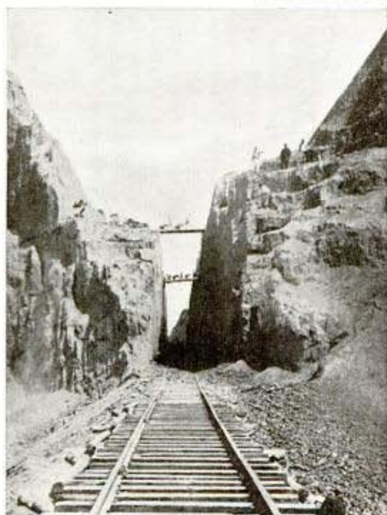
Track is laid in open tunnel cut through rock. Upper right, changing river's course to save building bridge
