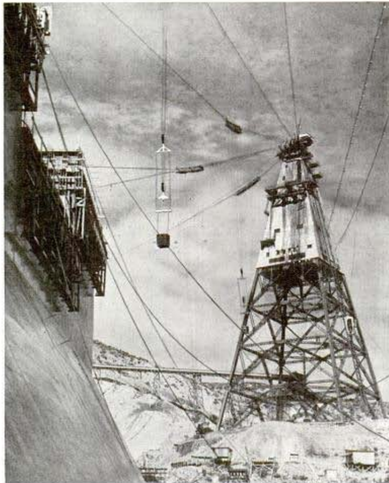
Each cableway bucket carries a 16-ton load of concrete to Shasta dam
