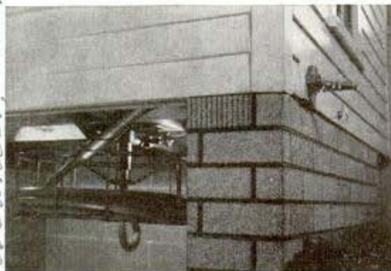
Hose reel on ceiling is connected direct to faucet
