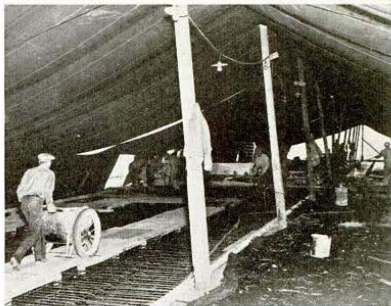
Tent on bridge (top) covered men (bottom) so they could work in all kinds of weather
