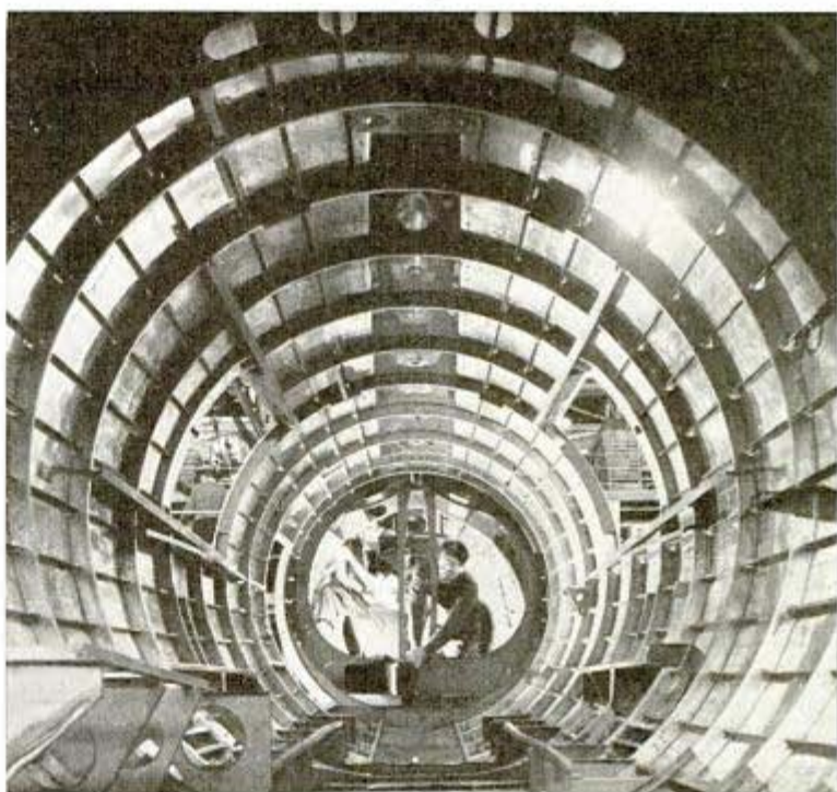
Looking aft in fuselage of a heavy bombing plane gives you some idea of what it takes to build a large all-metal ship like this one
