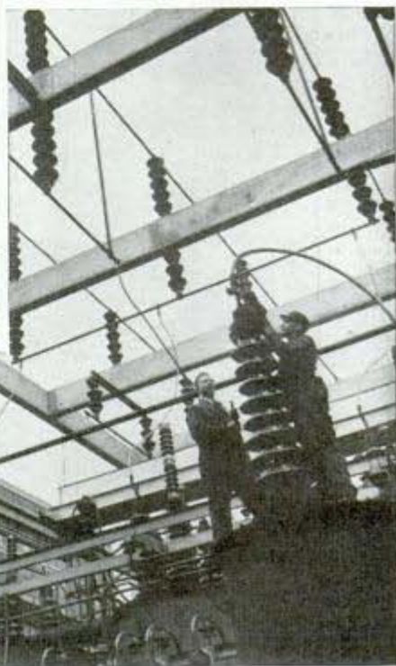
Bank of 15-foot transformers in Westinghouse high-voltage yard
