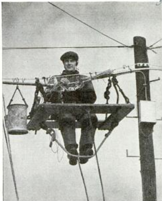
On outskirts of New York a lineman repairs one of the 200-pair cables which contains 400 wires
