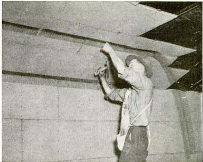
Wood fiber insulation board not only is protection against attic heat loss but also is good plaster base for walls of extra attic room
