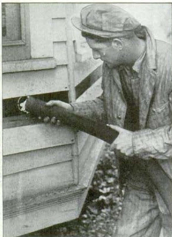
Blowing insulation into wall results in saving as much as 72.6 percent of the heat escaping there
