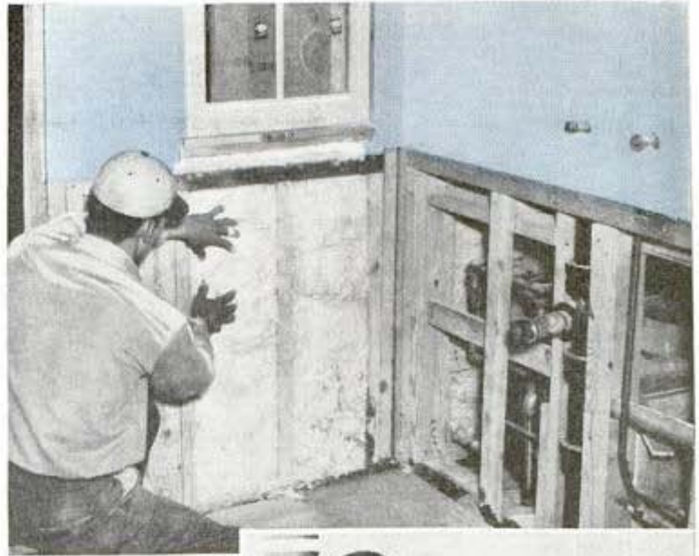
↑ Installing insulation in all-electric house; this work must be done properly to hold heating costs at reasonable levels
