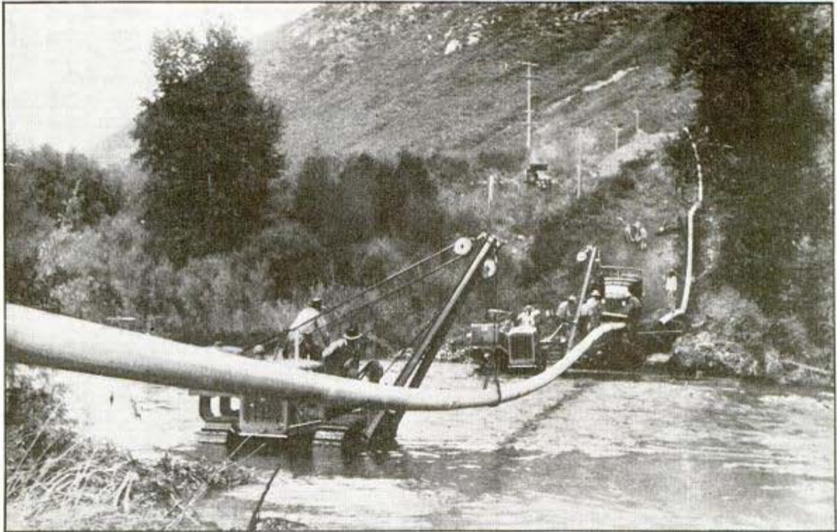
First pipe line to cross continental divide, from Wyoming to Salt Lake City, is lowered to river bed
