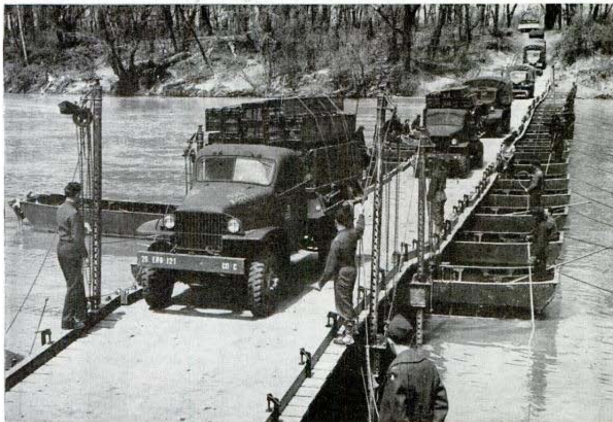
U. S. Engineers threw this pontoon bridge across Chattahoochee river in 41½ minutes. Front truck carries foot bridge units
