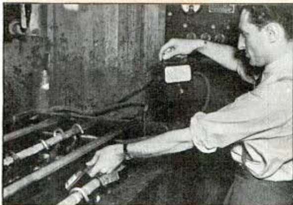
Velometer tests a tank of acid for surface ventilation as air is forced horizontally across surface
