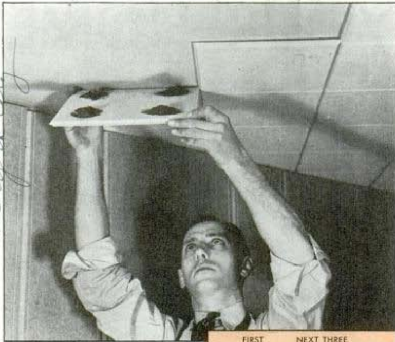
Insulating tile board may be applied to ceiling by using an adhesive
