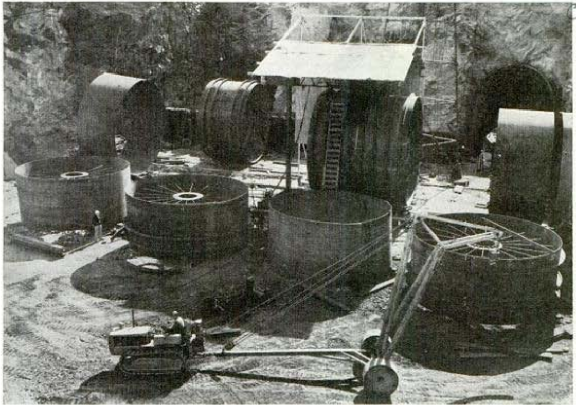
Large pipe many times their size is picked up and lowered into tunnel pit by tractor and trailer
